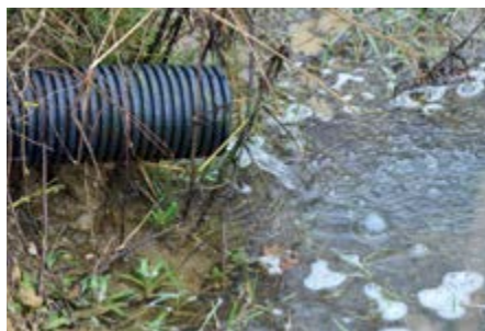
Drains should flow freely, and the water should be clear.
